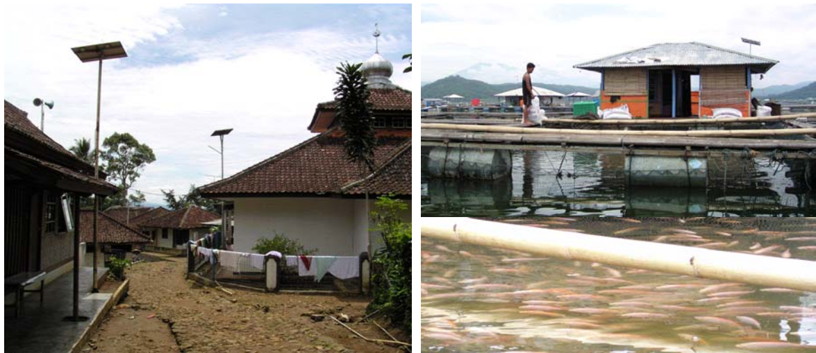
Figure 1a. (left) PV installations in Sukatani village, West Java, fifteen years after its inception. 1b. (right) PV systems installed on a hut roof of a fish floating net at Cirata dam, in the Jangari village, West Java.
