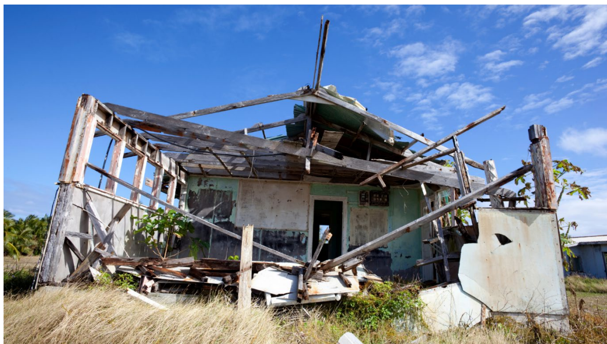
Figure 7: A cyclone-damaged building in the South Pacific
