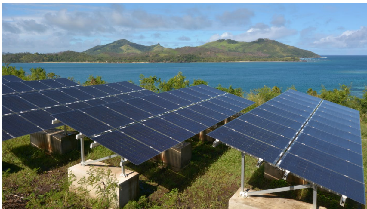
Figure 3: Ground-mount PV, Fiji
