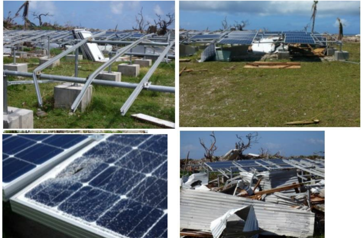
Cyclone Maysak Damage (FSM), SPC 2015
