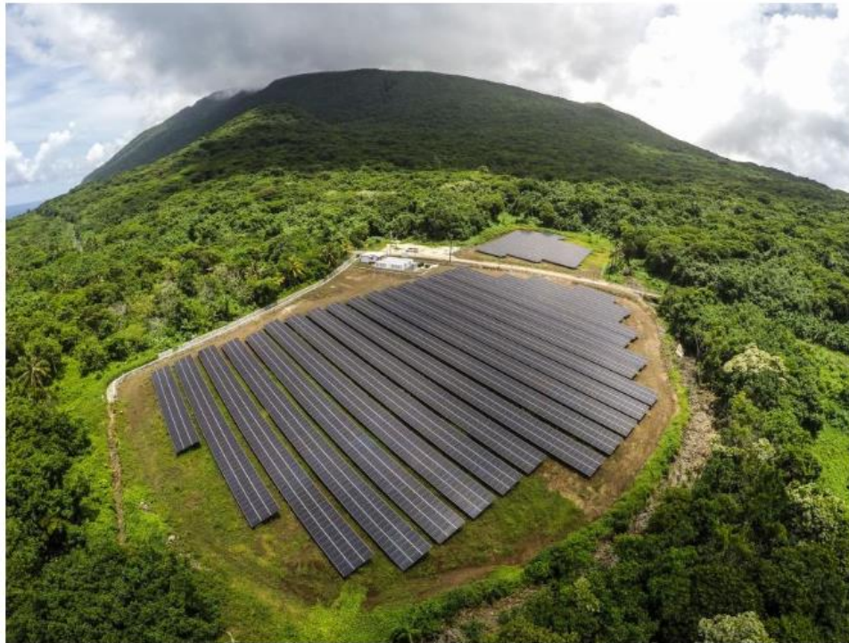
This seven-acre solar plant now provides all the power used on Ta'u Island.
